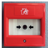
Fire alarm call point
