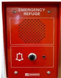
Commend refuge communications intercom
