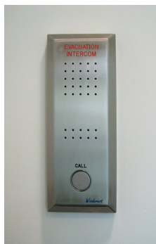
Windcrest refuge and lift communications intercom
