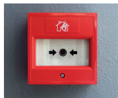
Fire alarm call point
