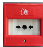
Fire alarm call point
