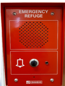
Commend refuge communications intercom
