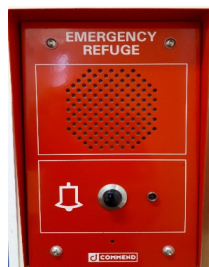
Commend refuge communications intercom
