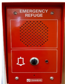
Commend refuge communications intercom
