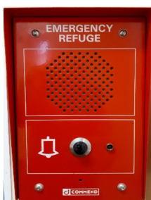
Commend refuge communications intercom
