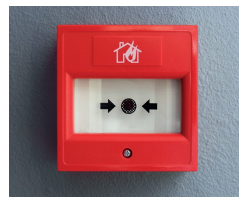
Fire alarm call point
